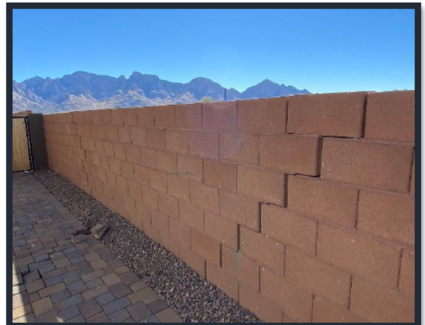
Figure 4: Lot 20 cracking observed in block wall and pavers at base of the privacy wall
