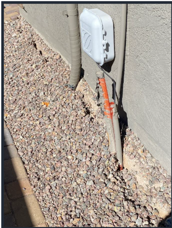
Figure 5: Lot 20 cracking of soil along base of the house
