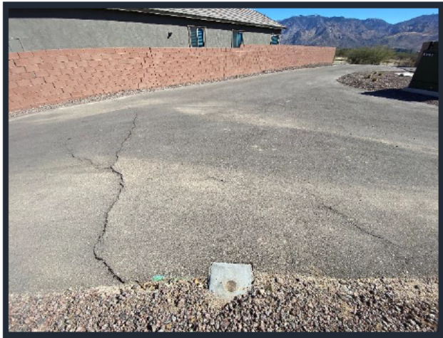
Figure 3: Cracking in common area of booster station, in the asphalt pavement, and leading to Lot 20. Similar residual cracking patterns in both wall and asphalt pavement
