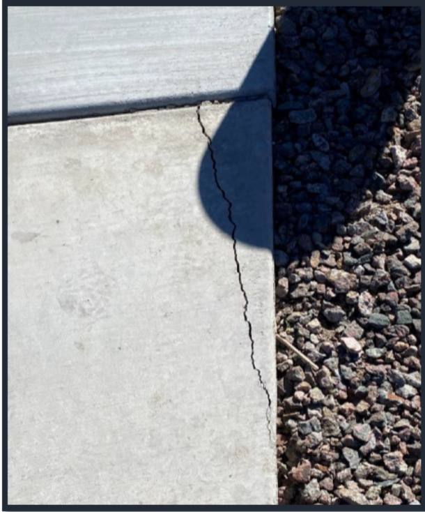
Figure 1: Lot 20, cracking in concrete driveway
